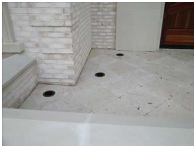
Apollo well lights were placed in custom-drilled holes in the entranceway's marble hardscape. The lights illuminate the brick surfaces on either side of the home's front door.
